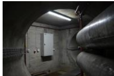
LED Röhren in Versorgungstunnel
